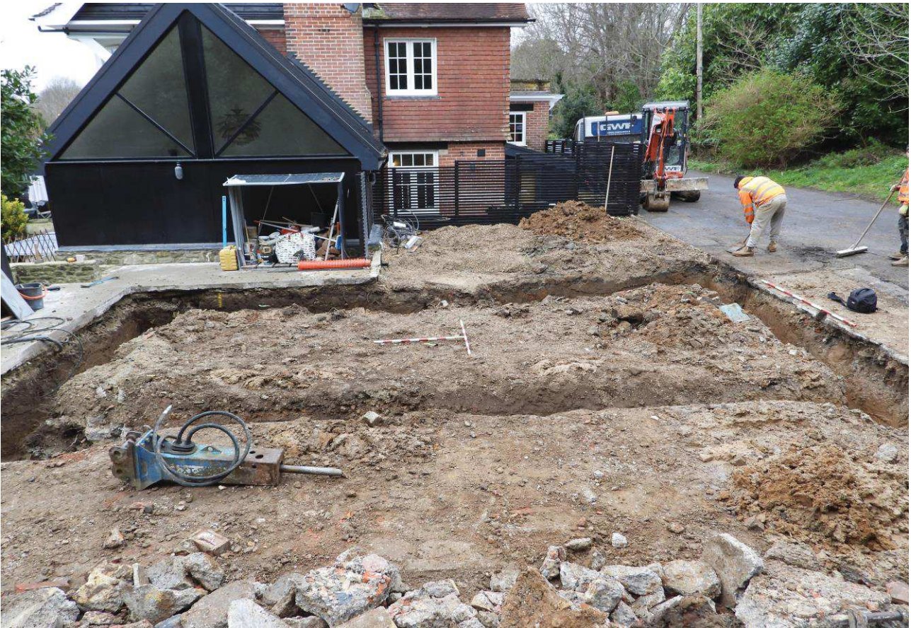
Plate 4: Foundation trench looking west with one-metre scales. Previously recorded 2019 excavation was located underneath black building (the extension).
