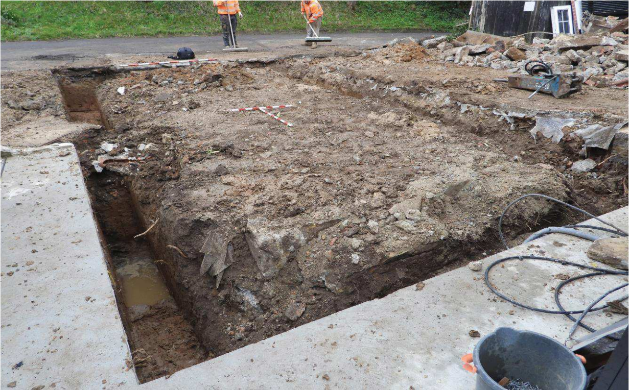
Plate 3: Foundation trench, looking south. Two one-metre scales and one two metre scale.
